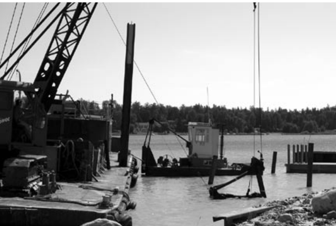
While dredging, MCM Excavating struggles to get the jaws around one of many huge boulders at the McKay Bay access site on Lake Huron.
