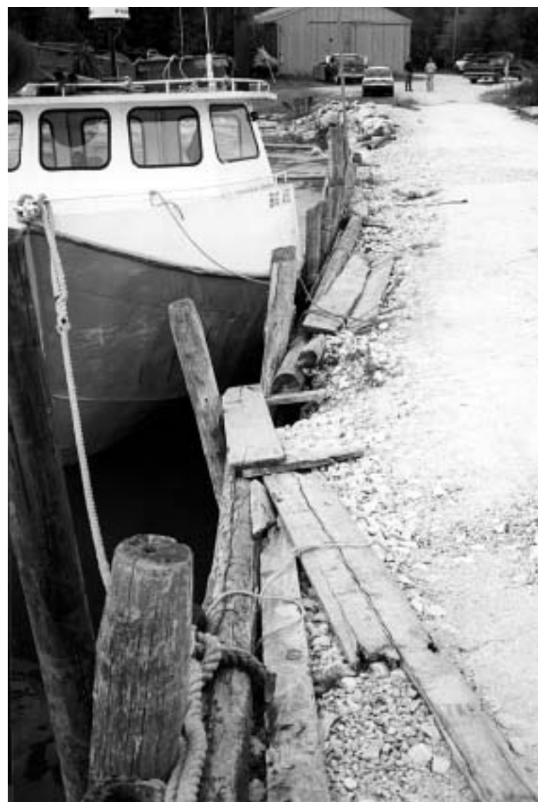
Existing docking and mooring facilities at Dutcher's are in need of repair.
